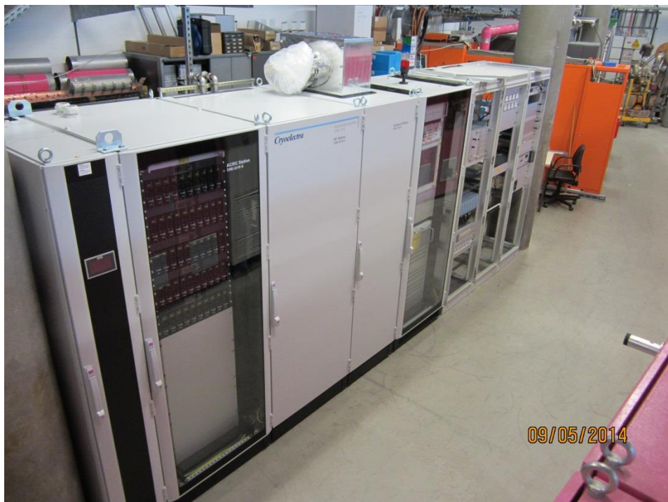
500 MHz 40 kW SSA transmitter by Cryoelectra
