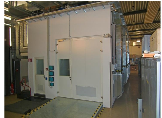
Clean room with HPR
