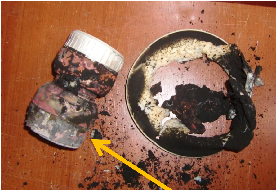
Burned contact springs of inner conductor
